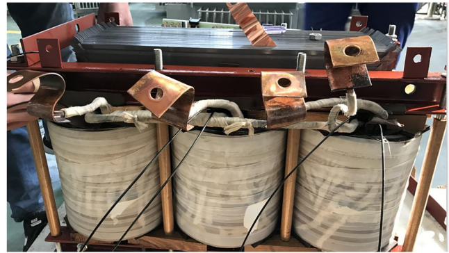
FIGURE 1 S13-M-100 kVA/10 kV transformer
