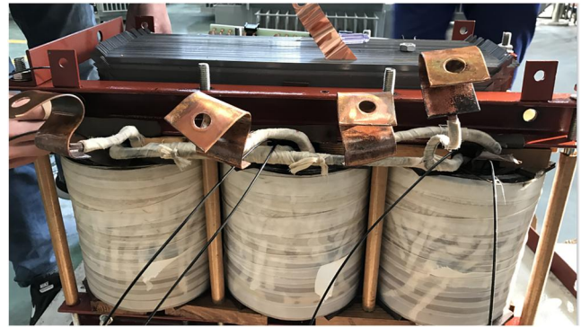
FIGURE 1 S13-M-100 kVA/10 kV transformer
