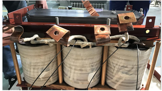
FIGURE 1 S13-M-100 kVA/10 kV transformer
